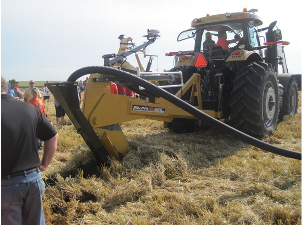
FIGURE 3. Ripping a trench at the Hefty Brothers' field day. (Photo courtesy of Frederick Errington)
